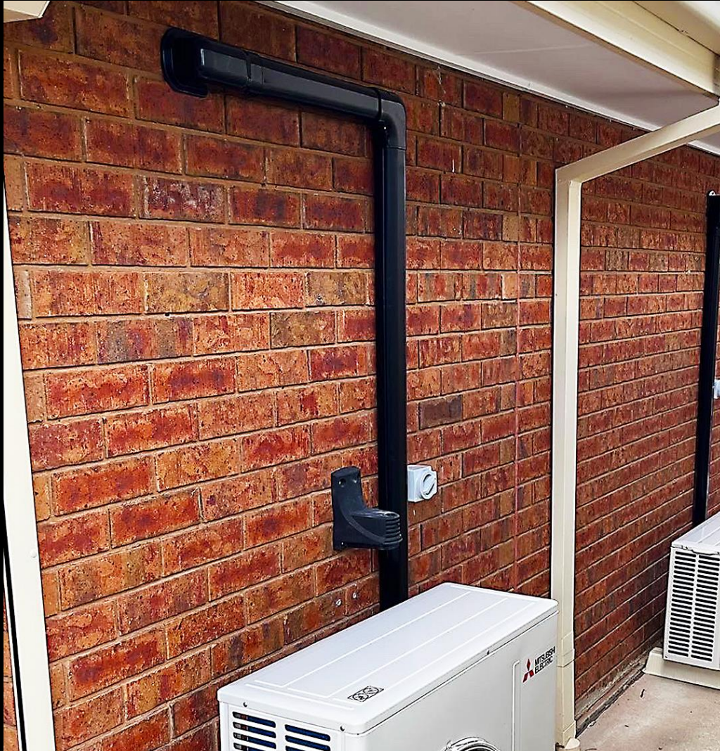
Installed by Dodds Heating & Cooling
