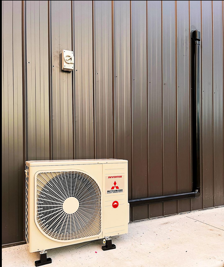
Installed by TEMPERCOOL AIR-CONDITIONING
