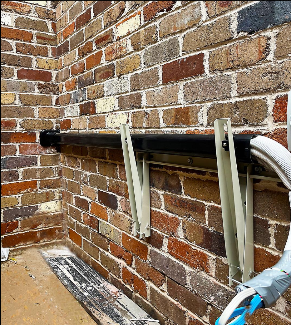
Installed by Premi air
