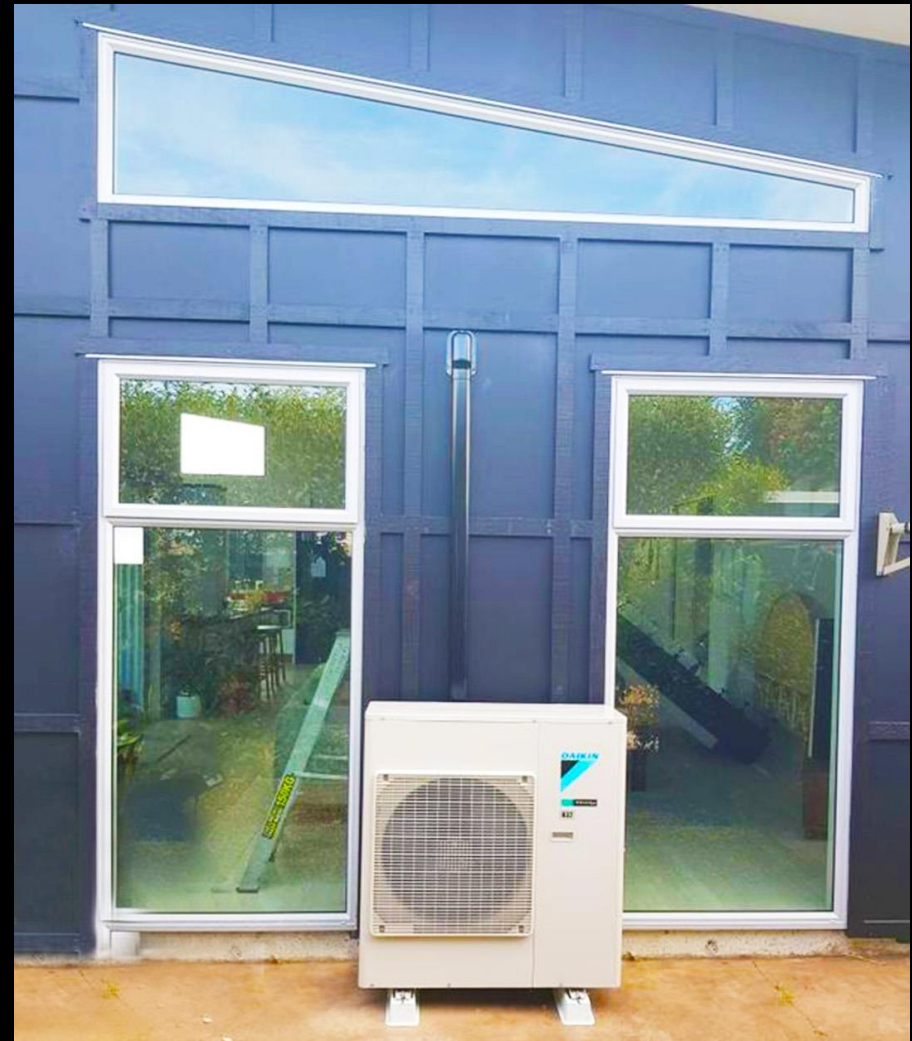
Installed by Cool wave
